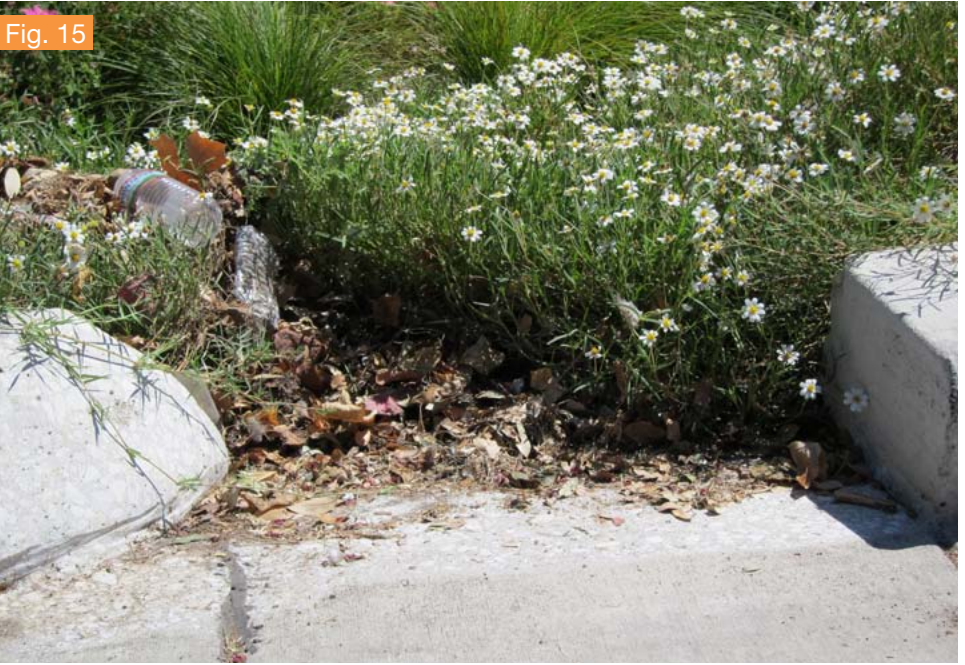
Curb inlet severely blocked by sediment and vegetation
