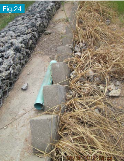
Level spreader clogged with sediment and debris
