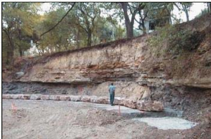
Erosion: West Bouldin Creek
