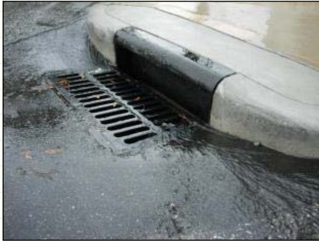
Stormwater enters inlet
